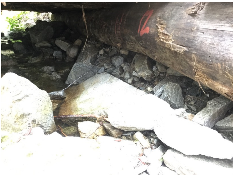
Downstream left bank sill scour
