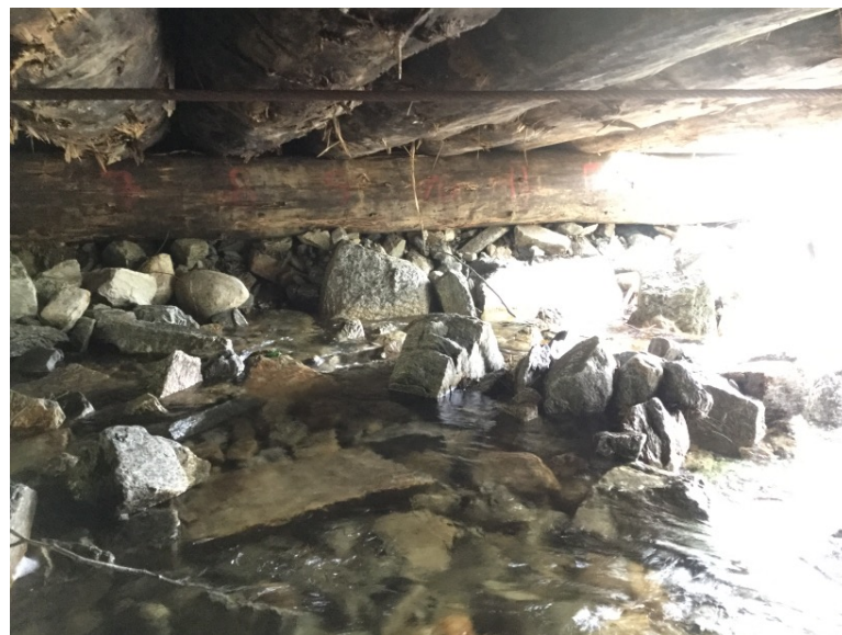
Downstream left bank starting to scour below sill
